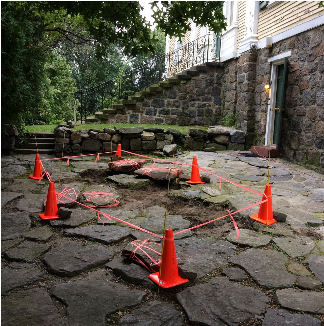
Figure 10- View of early excavation stage showing stone pavement (lower portion), rear entrance to house (right), terrace wall (center), terrace, and stairs above terrace (upper center).
